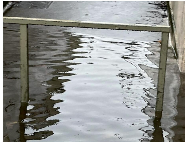
The flooded underpass in Rubery. Picture by Coun Esther Gray. s
