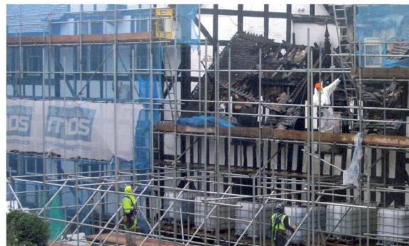
Work on the former Raven Hotel building which was devastated by fire in August. Picture by Paul Jones. 5
