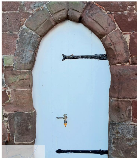
A 14th century wooden door at historic Peter Hall had a hole cut into it so a garden tap could be installed.
