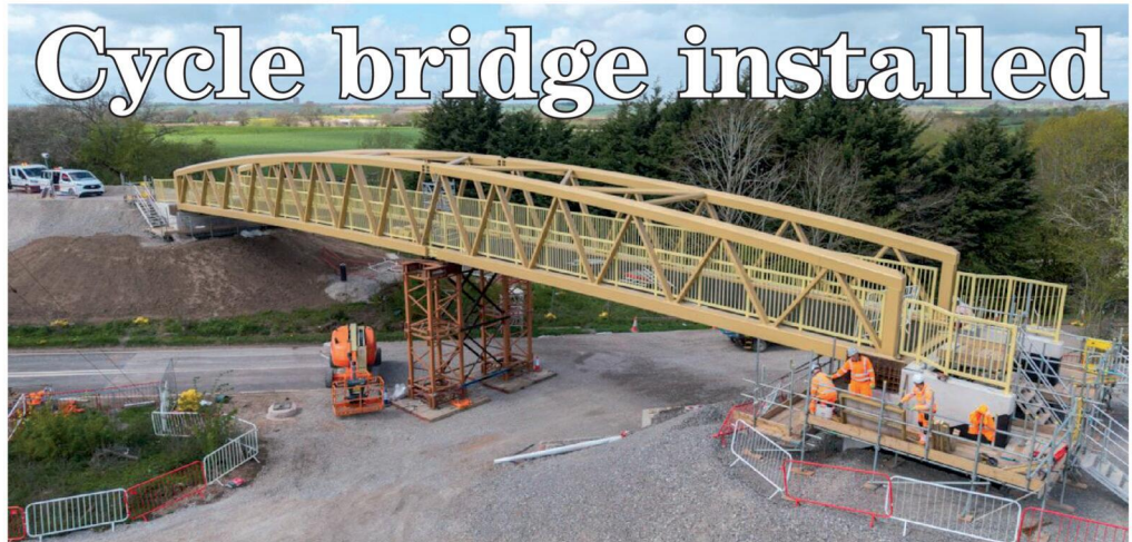
The new cycle bridge is in position over the Fosse Way. s
